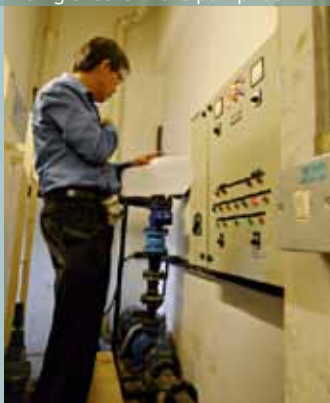
Doing checks in the pump room
